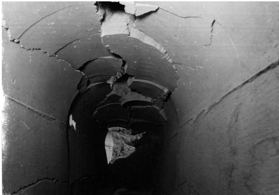
Figure 65. The results of the damage in Phase VIII.
